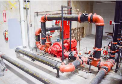
State of the Art Sprinkler System
